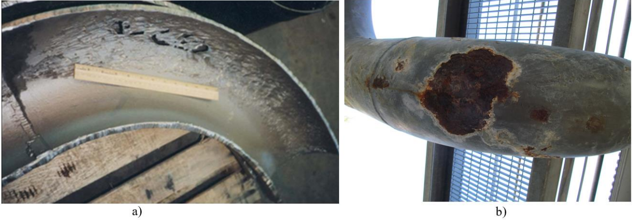
Fig. 1. Pipeline bends' defects: a) – erosion; b) – corrosion.
